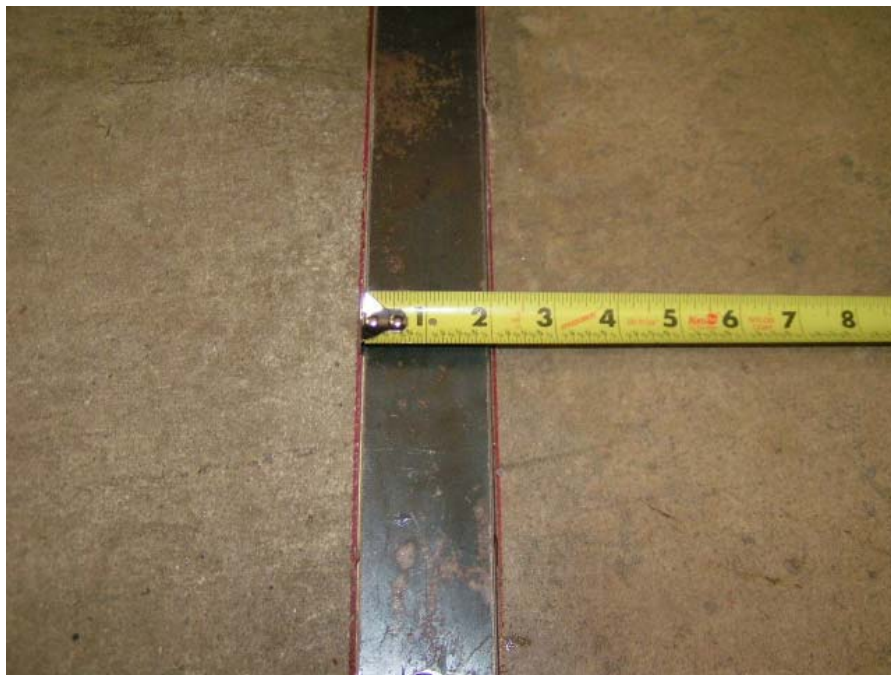
Photo 2: Steel Floor Hazard
